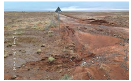
The damaged entrance to Keerweder after the November rainfall.
