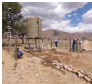
New water tank and fenced enclosure at Toekoms
