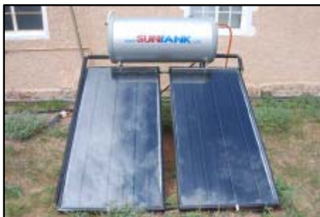
Toekom's new solar hot water heater
