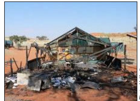
Main building after fire on 16 June.
